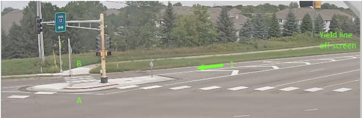
Figure 4-11 Site 1c in Burnsville at the northwest corner of TH-13 & Cliff Rd AFTER the installation of a flashing LED sign.
