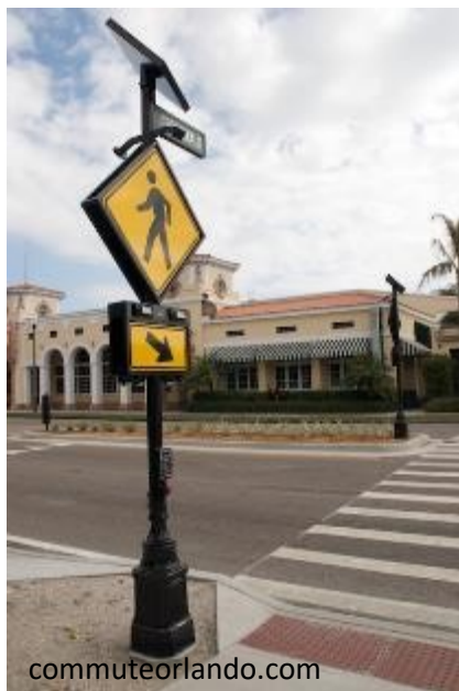
Figure 2-4 Example of RRFB (Photo courtesy of commuteorlando.com )
