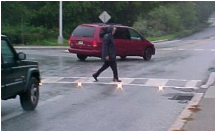
Figure 2-7 Example of in-pavement flashing warning light system
